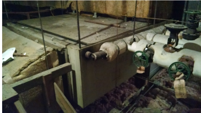
Figure 1 – Typical Air Handler Unit
