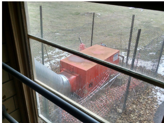
Figure 2 – Temporary Make-Up Air Unit
