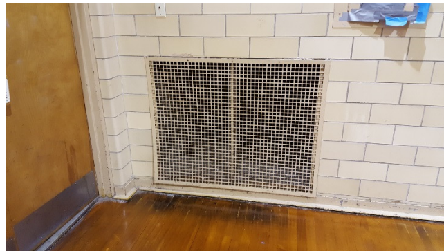
Figure 3 – Typical Gymnasium Exhaust Register
